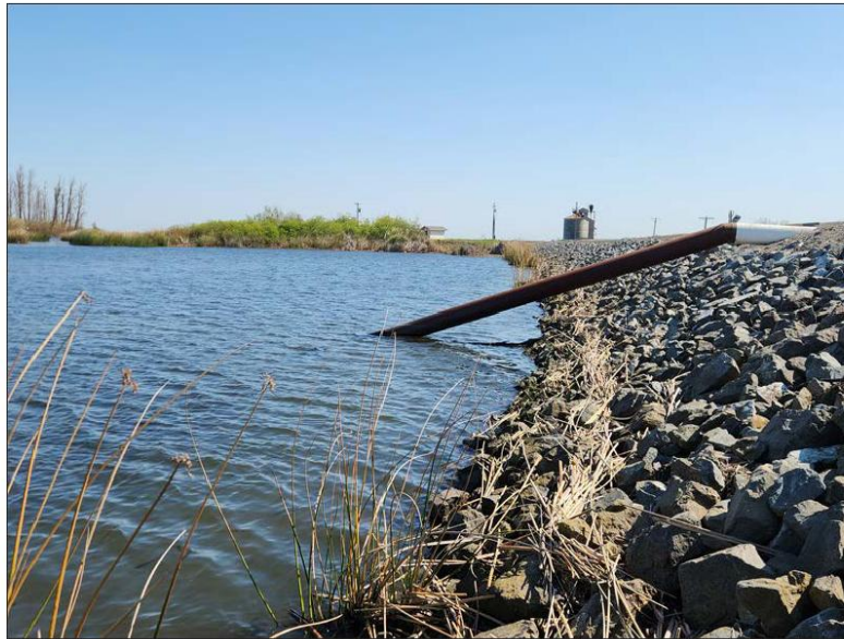
Photograph 7: View of the San Joaquin River with watermarks and drift deposits present on a pipe and along the levee. Photographer: Patrick Martin. Date: March 26, 2025.
